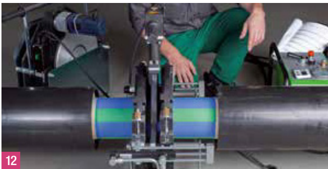
12 After the bead has achieved the preset height, the pressure is reduced at the hydraulic system. Then the heating up phase starts. Now the face sides in which the face sides of the pipe ends are heated up to the required welding temperature.
