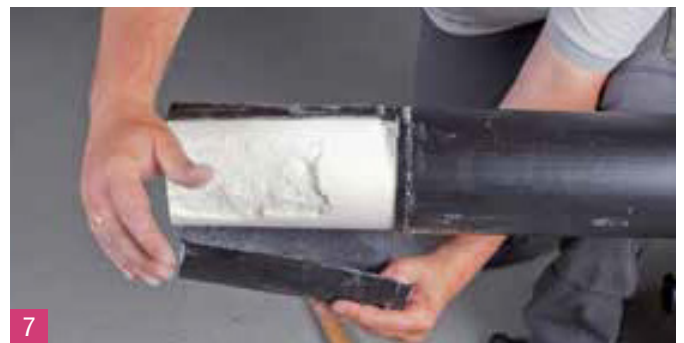
7 Detach the end of the casing pipe and then remove the PUR-insulation layer mechanically on the full skinning length.
