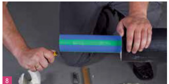
8 Clean the skinned medium pipe and deburr the pipe ends inside and outside.
