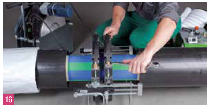
16 After the end of the cooling period the pressure is released at the hydraulic system. Then the mounting clamps are disconnected and the clamping device is removed.
