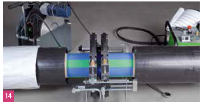
14 By using the hydraulic system the pipe ends are joined slowly until the required welding pressure is achieved.
